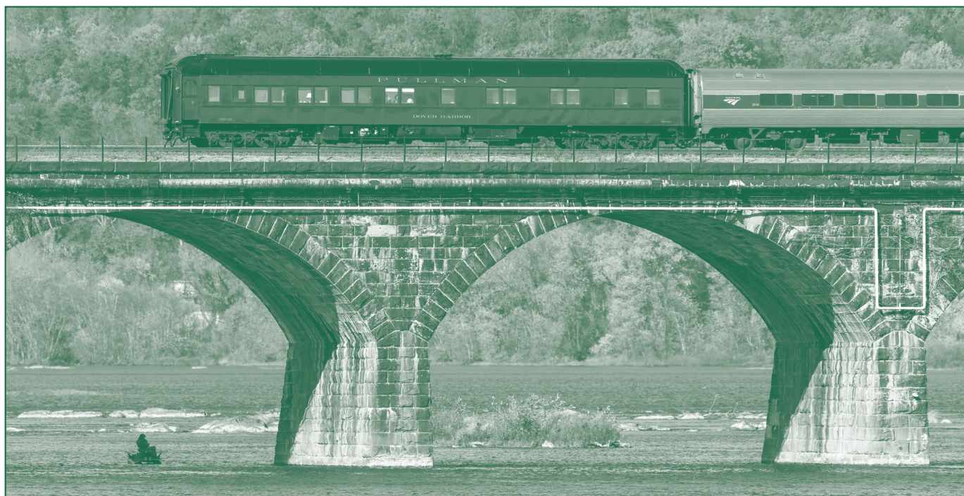
Traveling across Pennsylvania to New York, Dover Harbor crosses over the Susquehanna River on Rockville Bridge; photo by Rick Moyer.
